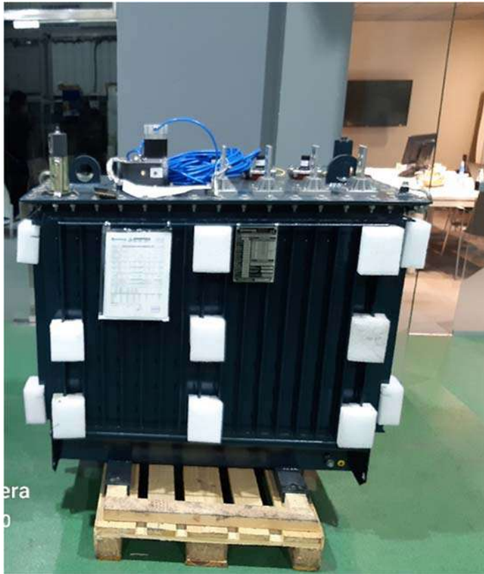
Figure 2: Smart trafo designed for Flexigrid
